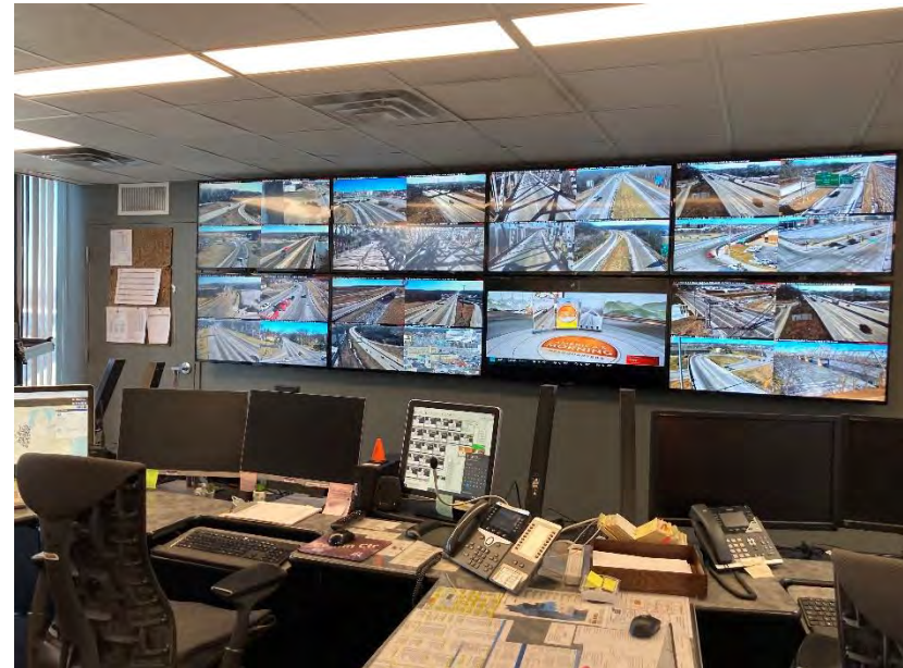
Figure 111: IDOT District 4 Communications Center in Downtown Peoria
